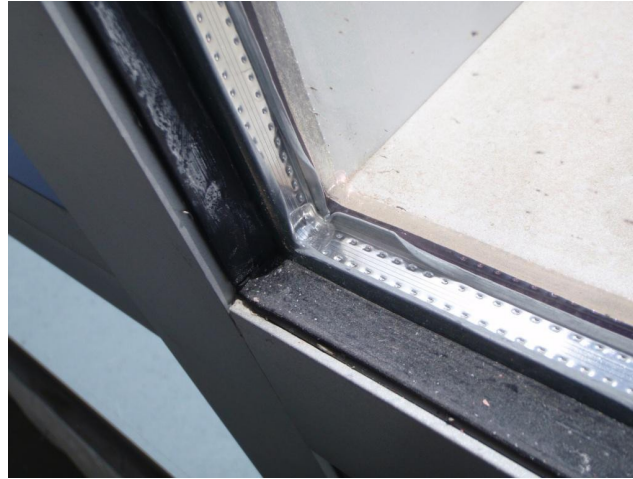
Figure 7 An Example of Primary Sealant Infringement
