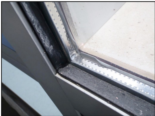
Figure 5 Primary Sealant at Desiccant Hole Location
